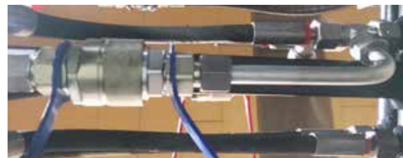
Fig. 63. Connected blue hydraulic hose
